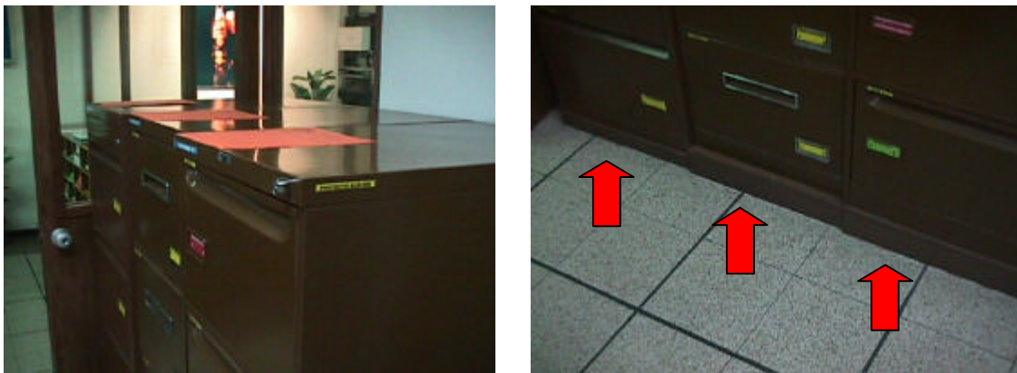
Fig. 5. Different cabinets are vertically aligned using wood wedges or blocks of different heights.
